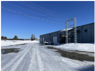
Site connection to hydro-power and major infrastructure
